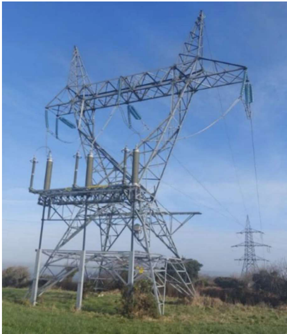
Figure 5.11: Line Cable Interface Mast (LCIM)
