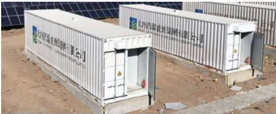
Figure 5.3: Image of a typical container housing the battery storage modules
